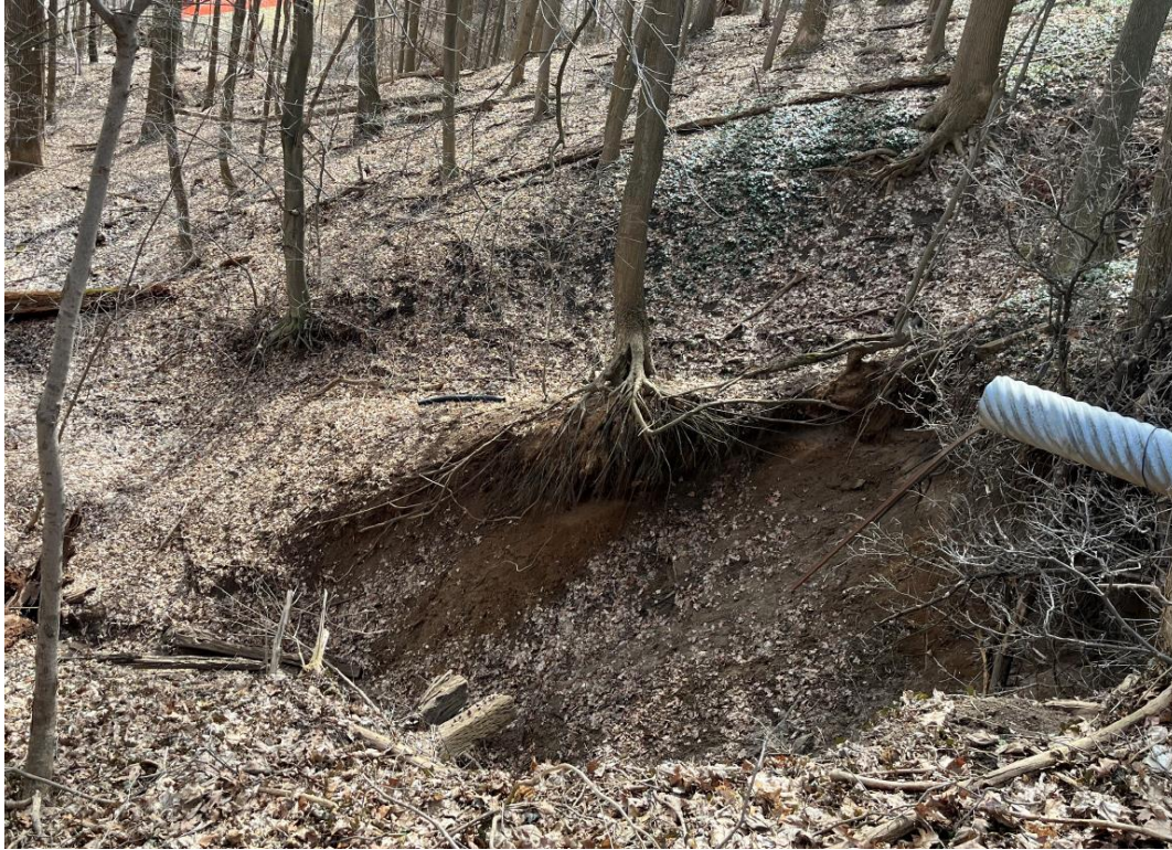
Spencer Lane Slope Failure, overlooking Marlene Stewart Park
