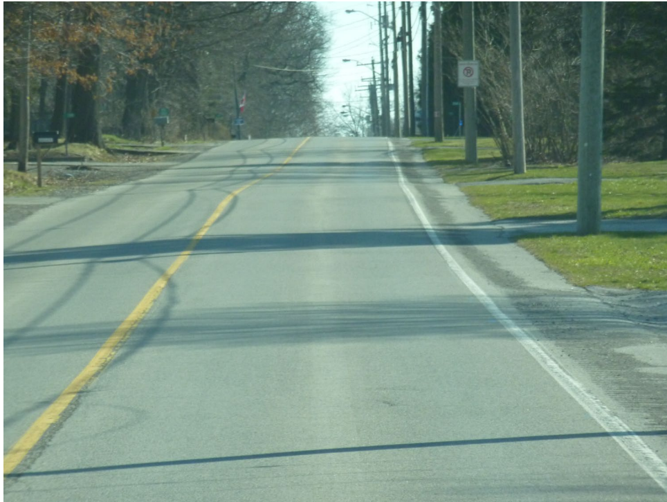
Figure 2-3. Section 420.07, Canboro Road, from Effingham Street to Oakridge Boulevard – HCB (Good Condition, PCI = 72)
