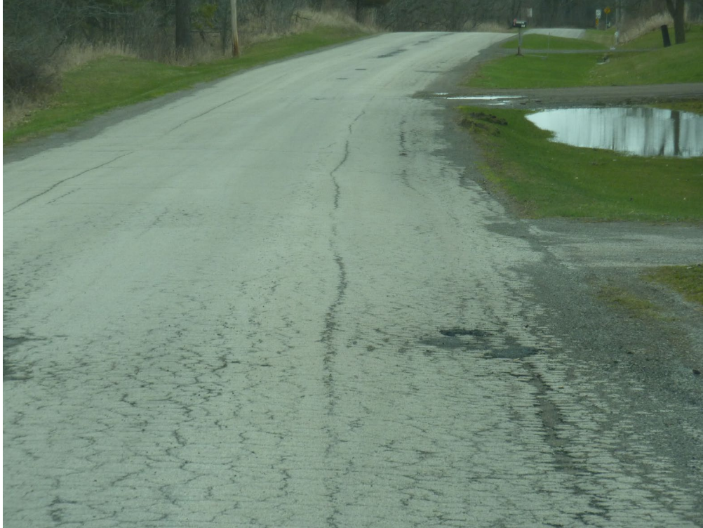
Figure 2-7. Section 114.06, Roland Road, from Effingham Street to Sulphur Springs Drive – LCB (Fair Condition, PCI = 54)
