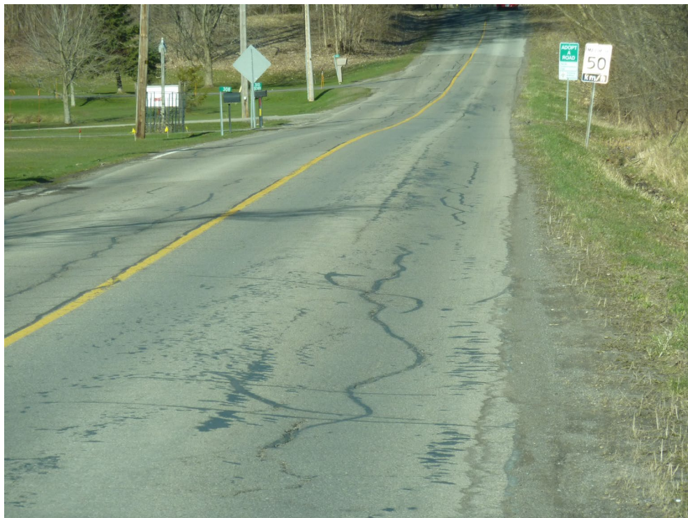
Figure 2-4. Section 206.06, Welland Road, from Centre Street to Effingham Street – HCB (Fair Condition, PCI = 56)
