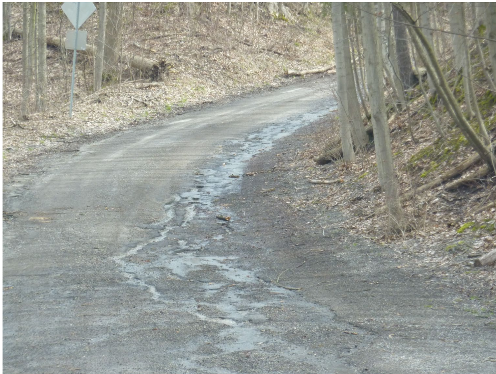
Figure 2-8. Section 121.01, Luffman Drive, from Sulphur Spring Drive to Orchard Hill Road – LCB (Poor Condition, PCI = 46)
