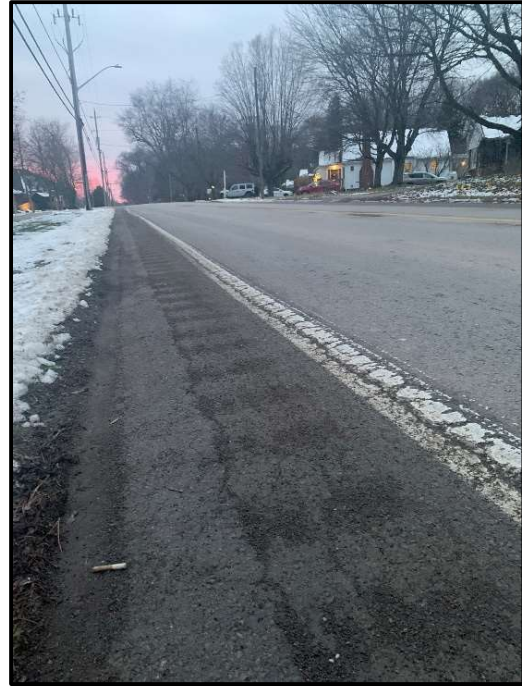
Figure 3.4 – Eroded Rumble Strips
