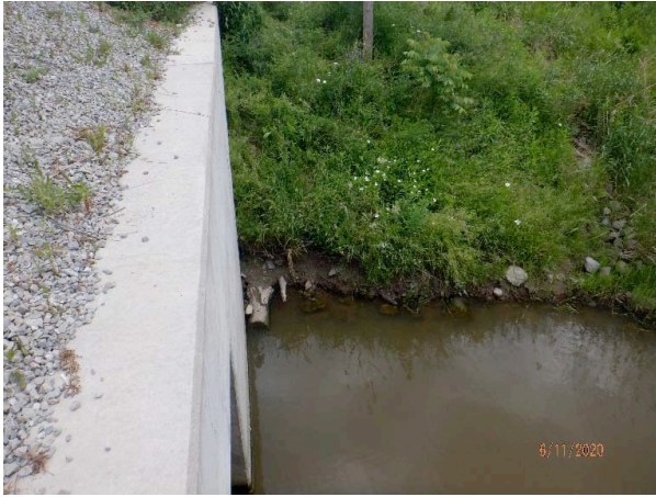
Figure 29. Erosion at southeast corner.
