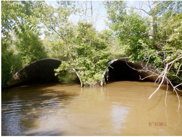
Figure 23. East end of pipes.
