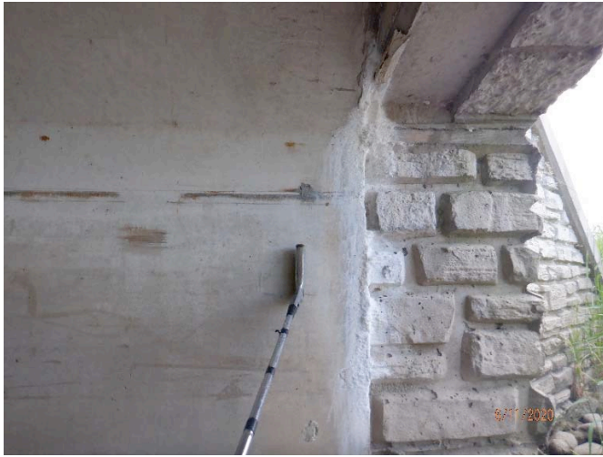
Figure 20. Leakage and efflorescent staining at northwest corner.
