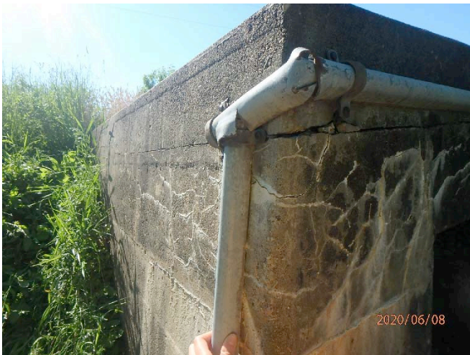
Figure 16. Wide horizontal crack at south east corner.
