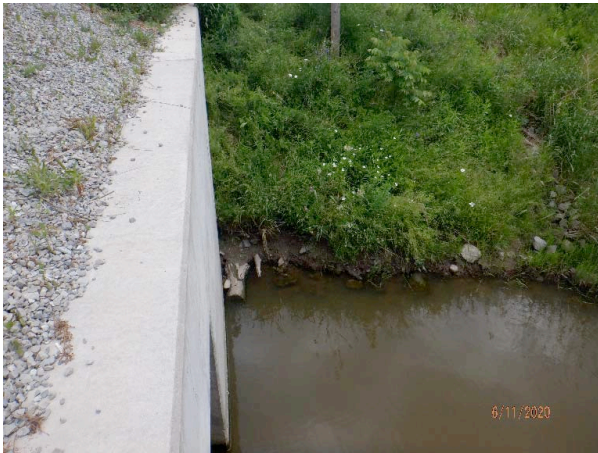
Figure 29. Erosion at southeast corner.
