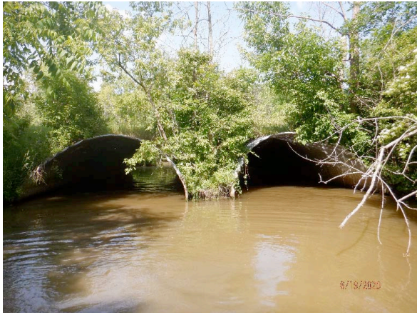
Figure 23. East end of pipes.
